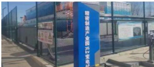
Zhangmu Town 35kV Substation
