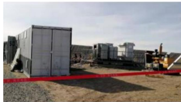
Engineering switchgear for Banyun Xian Wind Farm
