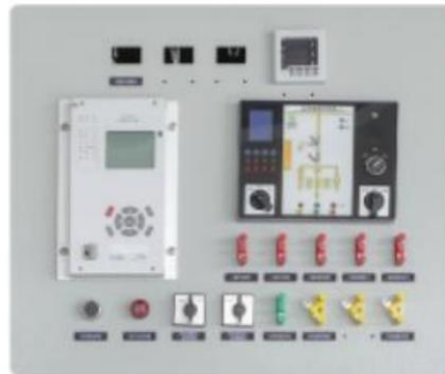
Secondary control room
