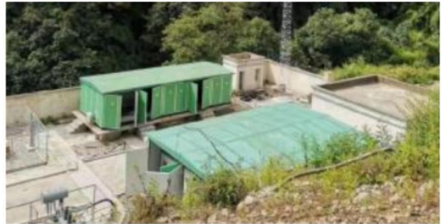
35kV transmission and transformation project in Aksu Muhu, Xinjiang
