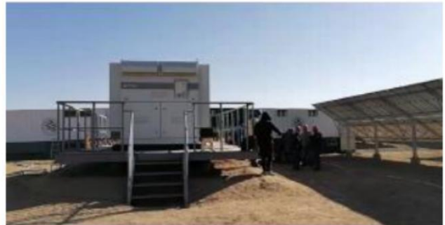
Complete set of power equipment for the Sichuan Tibet Railway
