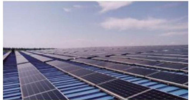
1600 MW Photovoltaic Project at the New Energy Base (One Zone, Two Parks) in Nanhai Prefecture, Qinghai Province
