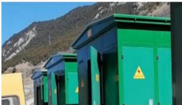
Central heating renovation (coal to electricity) 110kV substation project for Maqu county
