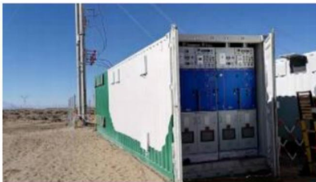
35kV gas charging cabinet for Guojiawan 110KV substation project
